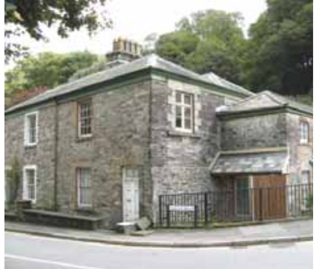
This listed house in Dolvin Road is vacant and in need of repairs
