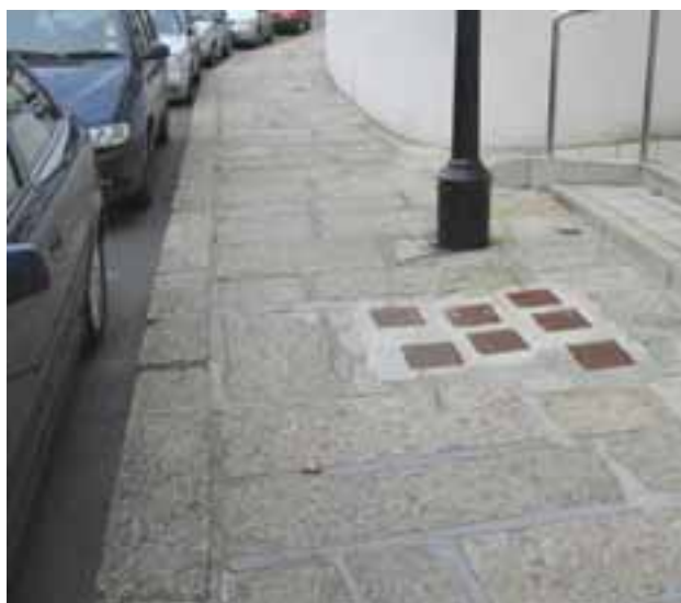
This section of historic granite paving in Russell Street has been adversely affected by the insertion of water meter covers
