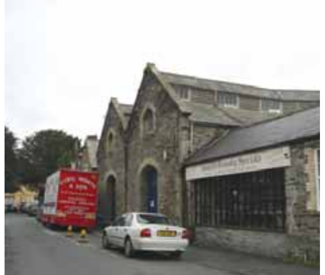
The Auction Rooms are in need of repair
