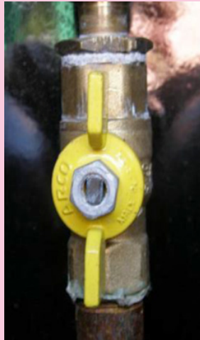
Emergency Control Valve
