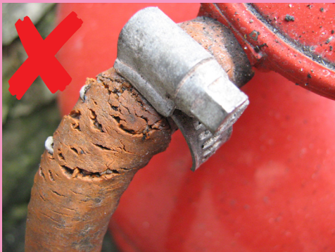
The pipe is badly cracked at the join and is likely to leak gas. Replace immediately.
