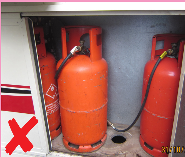
Holes have been made in the bottom of the cylinder compartment for ventilation. The cylinders are also not secure during transit.
