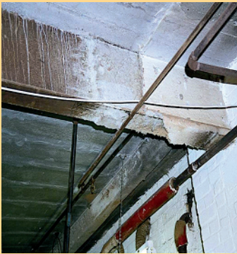
Sprayed Asbestos and Lagging.
